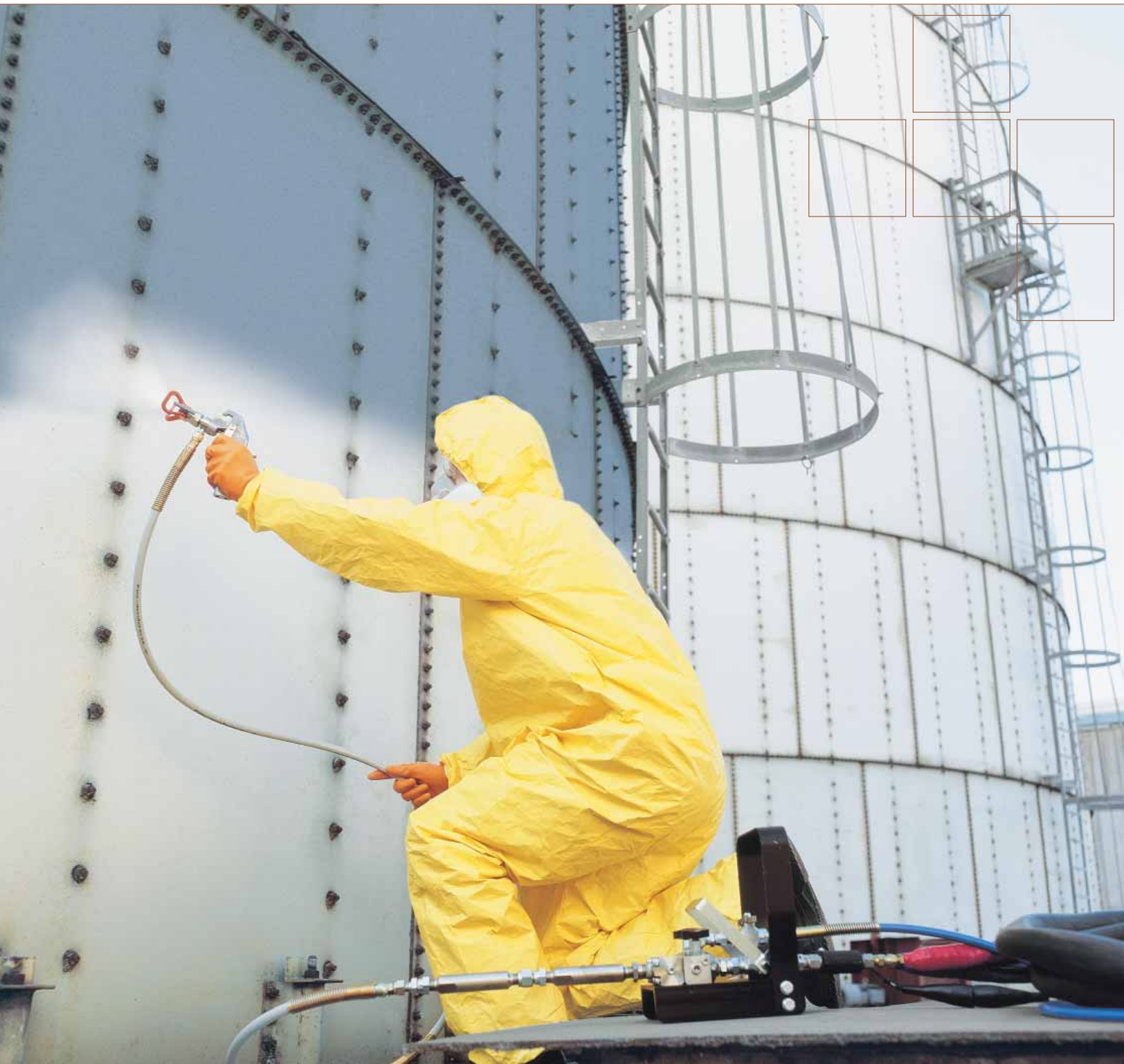
Quick-set plural-component spraying equipment with remote manifold is used to apply the latest hybrid coatings
